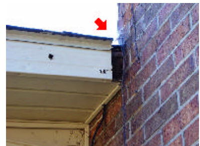
Attic view of porch roof leak
